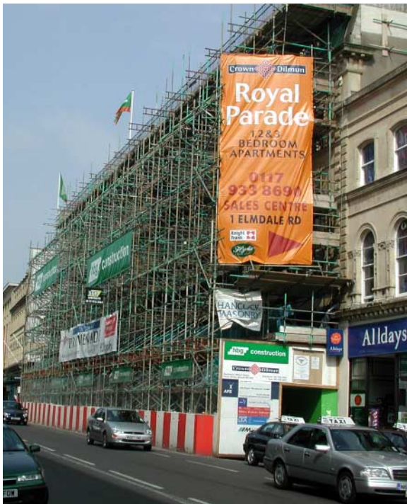
Current scheme in progress. The conversion of the former Dingles store on Queen's Road, Clifton by Crown Dilmum has secured on-site affordable housing provision
