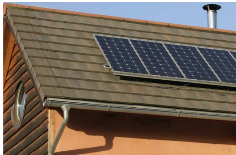
Use of solar panels on a new house in Ashley Vale.
