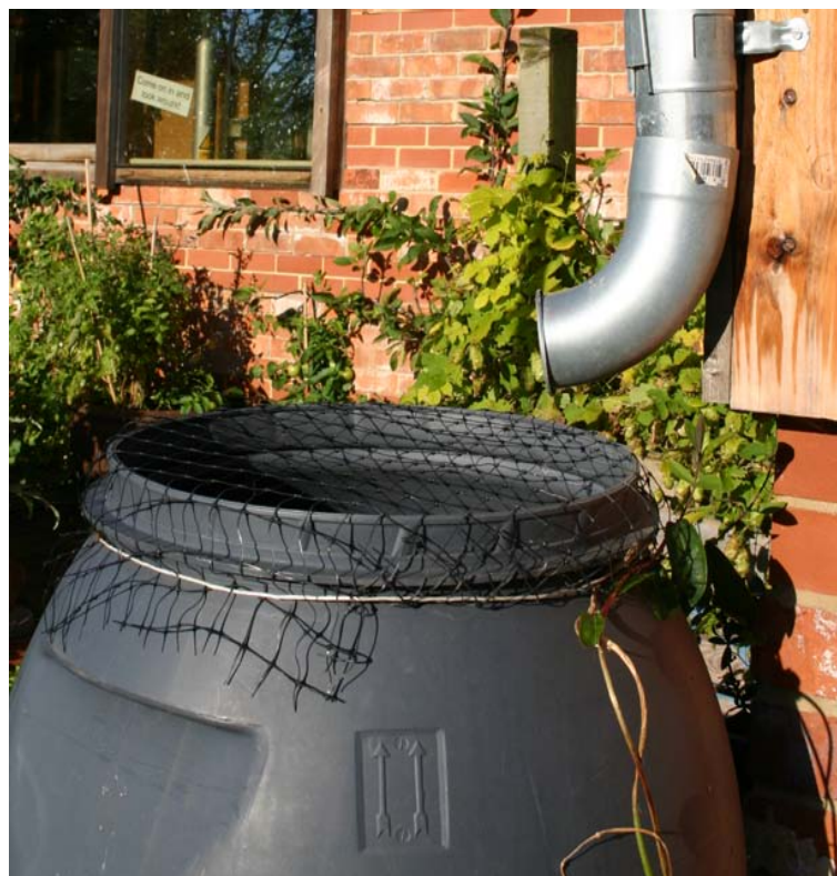
Using water butts to collect rainwater is a simple low cost measure.
