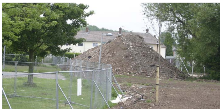
Some of the rubble generated by the demolition of Henbury School ready to be re-used.
