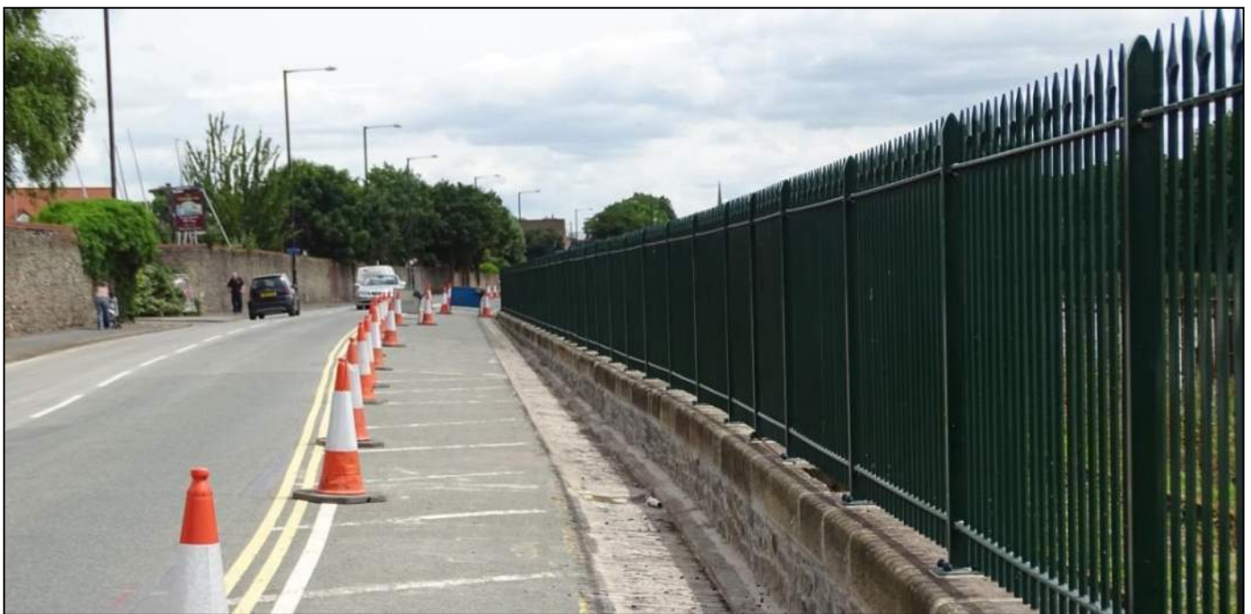
Figure 21: The MetroBus flood wall on Cumberland Road
