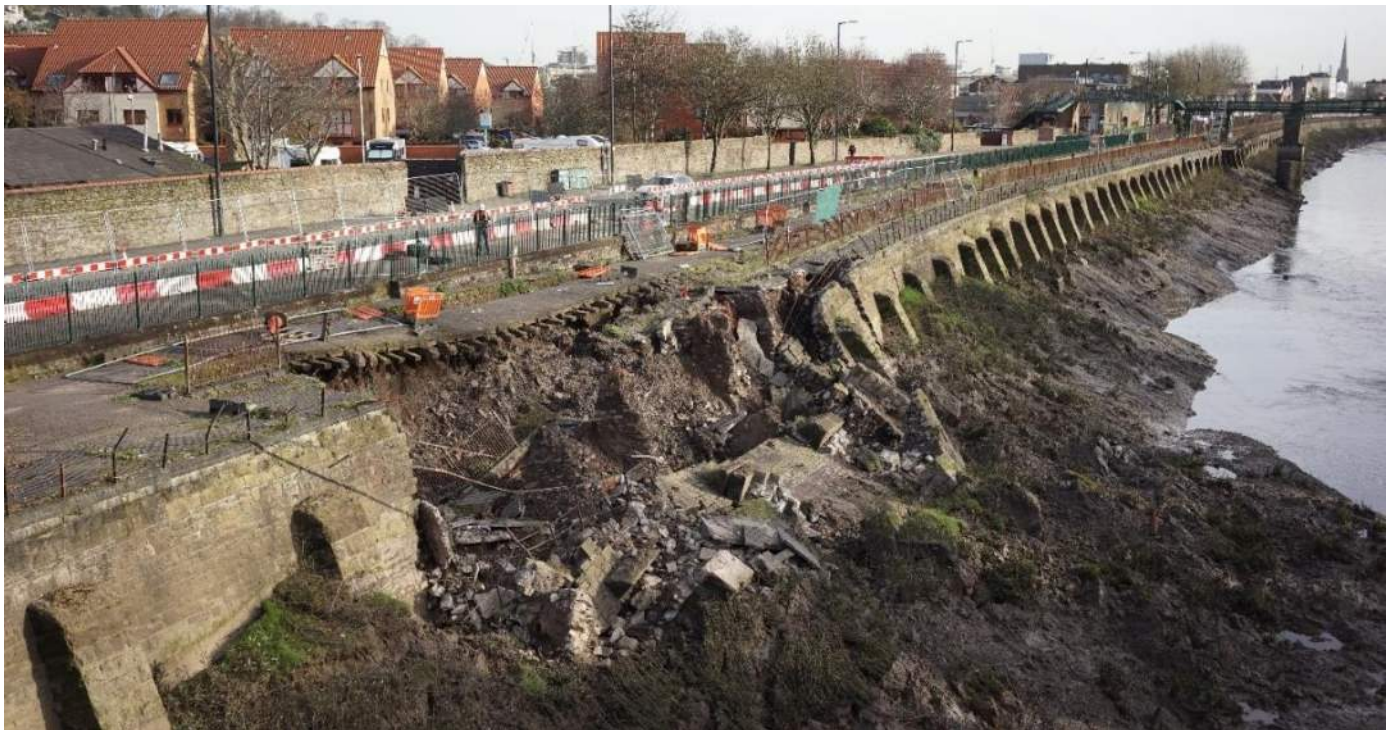
Figure 23: Photo showing the collapse of the riparian wall on Cumberland Road in 2019
