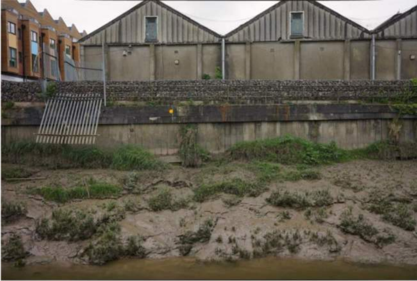
Figure 3: Images of flood wall asset NCS41(taken from the information provided by BCC).
