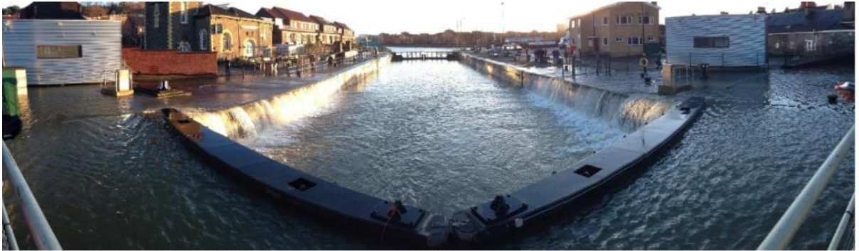
Picture 1: Flood flows bypassing the lock gates.
