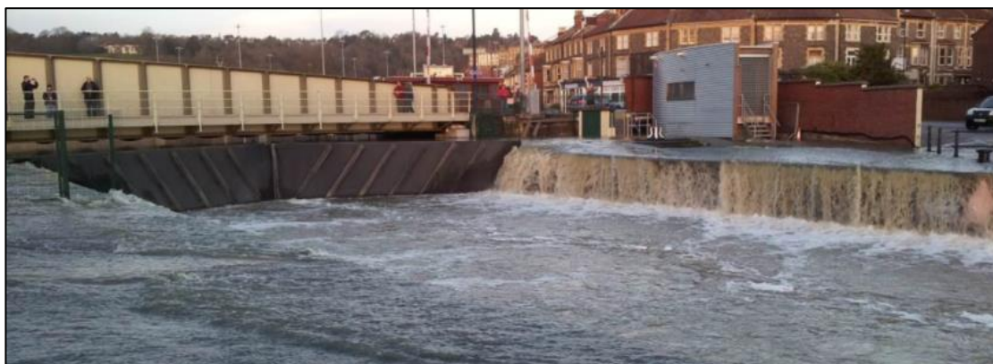
Figure 3. Photograph showing Cumberland Basin overflowing into the Floating Harbour at Junction Lock, 2014 (phot from the first phase feasibility study)
