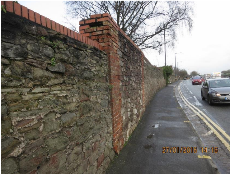
Figure 6 - Photo of the wall taken between the entrance to Underhill Yard and Cottage Inn car parks
