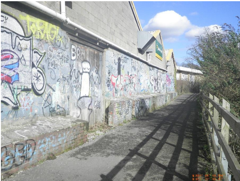
Figure 33 - Example of a wall considered to be condition grade 4
