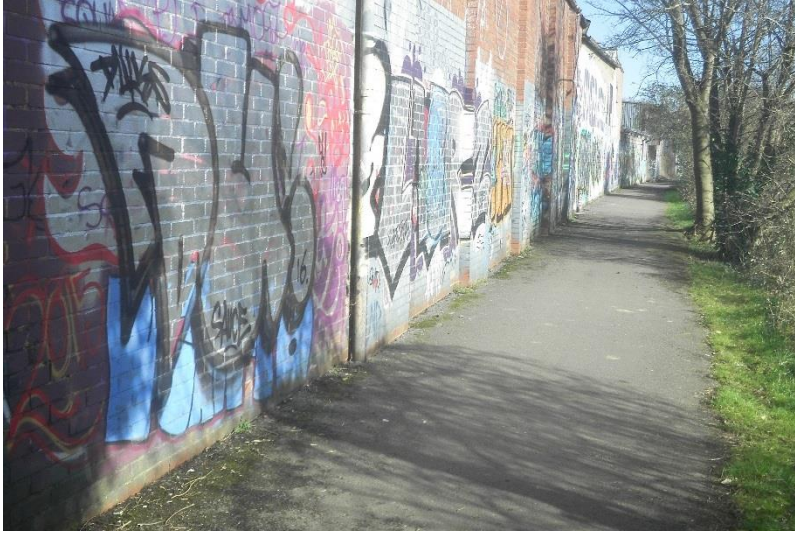
Figure 32 - Example of a wall considered to be condition grade 2
