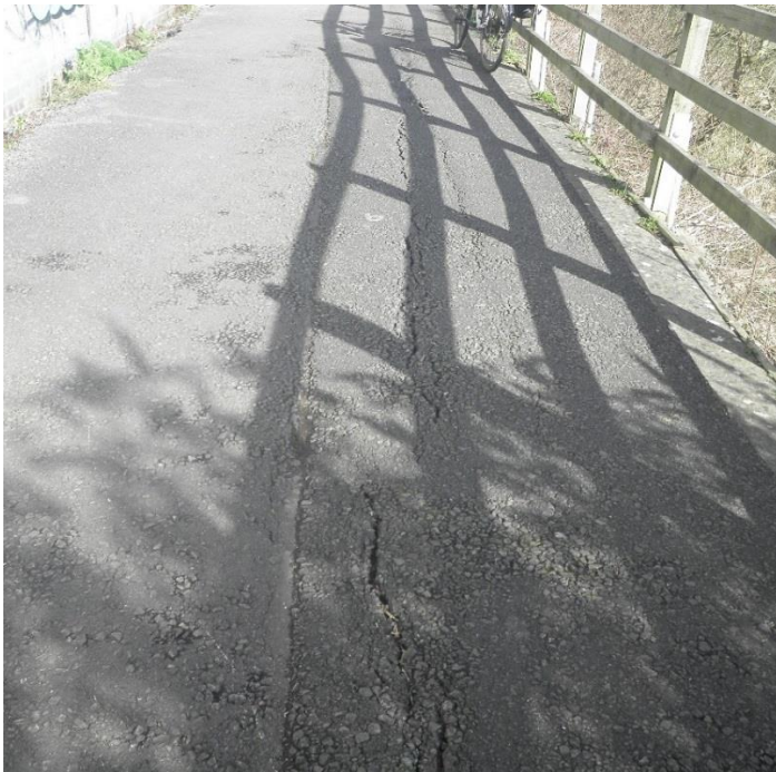
Figure 37 - Cracks in path
