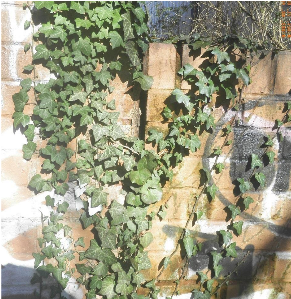
Figure 34 - Wall marked *, condition grade 4
