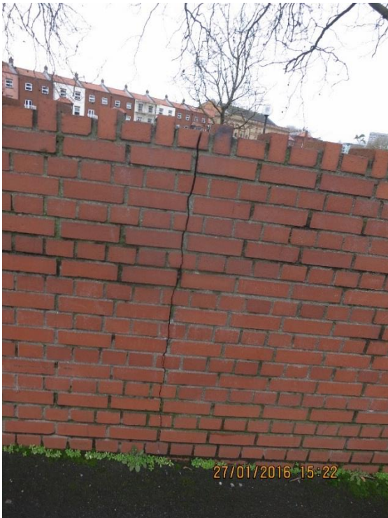
Figure 11 – typical vertical crack in the wall
