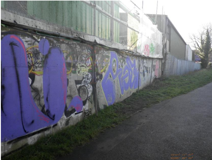
Figure 22 - Concrete wall, the tie in to the embankment can be seen on the right
