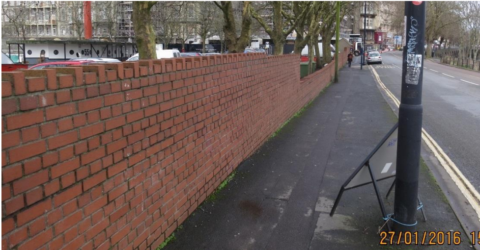
Figure 10 - Photo taken near the west end of the wall, looking east. The railing on the right of the road are on the alignment of the Environment Agency's definition of top of the bank.
