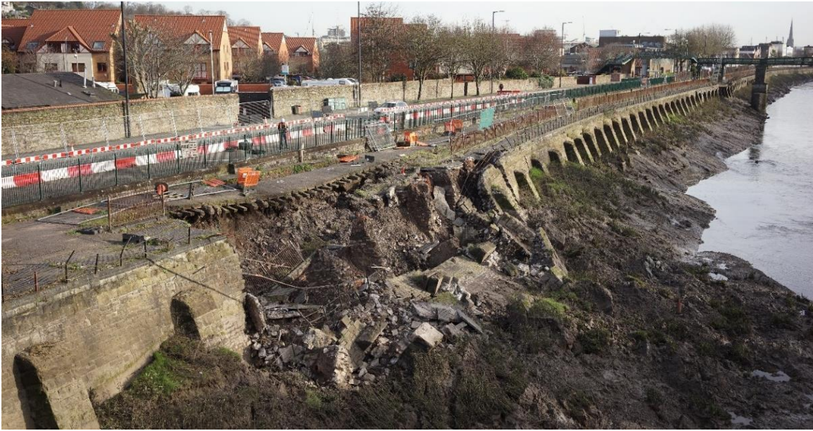
Figure 7: Showing the historic 2019 slip on Cumberland Road
