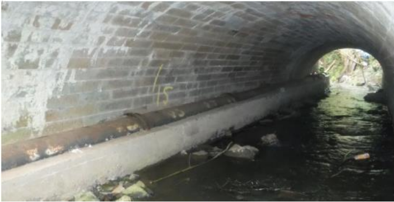
Figure 10: Concrete encased service pipe within the Network Rail culvert (photo taken on 24/04/2019).
