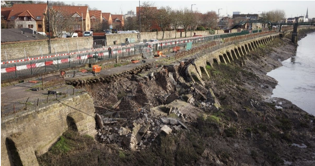
Picture 1: Collapse of the riparian wall on Cumberland Road in 2020
