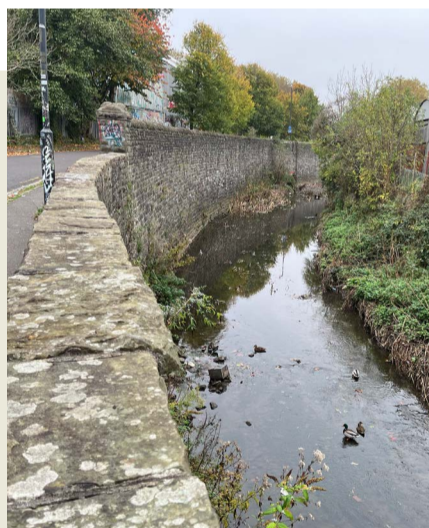
Litter and debris affect the existing water quality.
