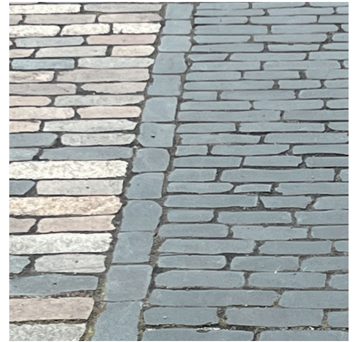
Projects elsewhere in Bristol city centre have demonstrated that historic sett surfaces can be retained whilst significantly boosting accessibility.
