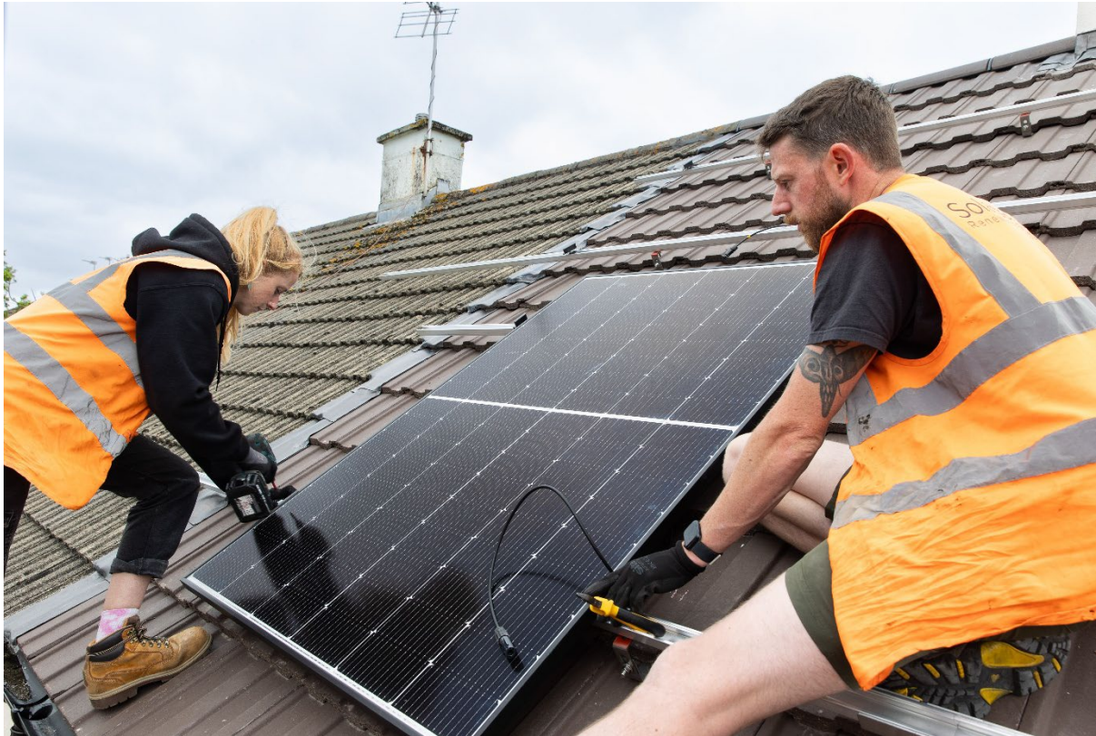
Figure 22: Two people installing solar panels on a Bristol City Council home in Brentry. Image credit: West of England Mayoral Combined Authority.
