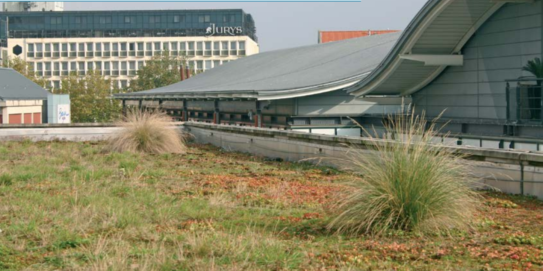
At-Bristol Centre green roof retrofitted onto an existing flat concrete roof in 1999
