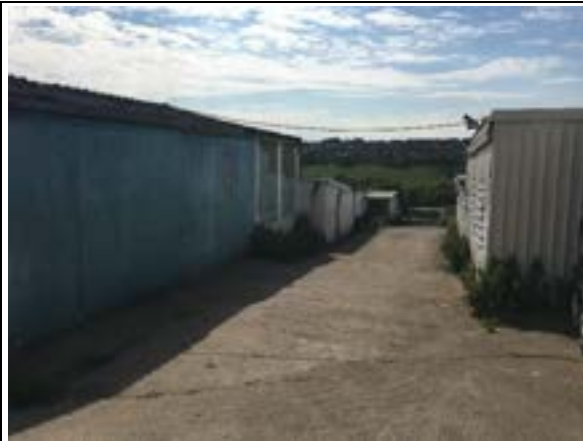
Photo 1: Stable buildings with low bat roost suitability where a re-entry survey took place.
