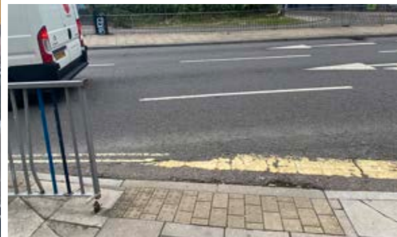
Tactiles indicate crossing where no crossing exists
